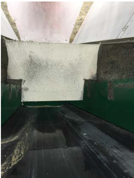
ABOVE: After image showing the installation of the product combination, outside and inside the chute. RIGHT: Video of effective transfer point in action >> CLICK VIEW
