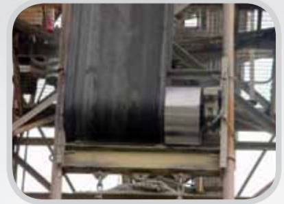
A typical mistracking problem resulting in product spillage and possible damage to the belt, mechanical splices and/or conveyor structure.
