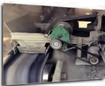
Belt conveyor drive
